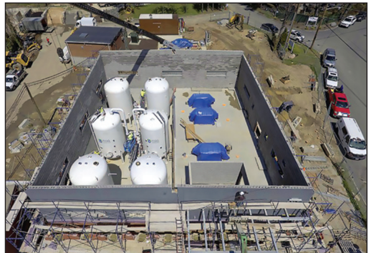
These drone photos show the project at its early stage (top) and more recently (bottom).
