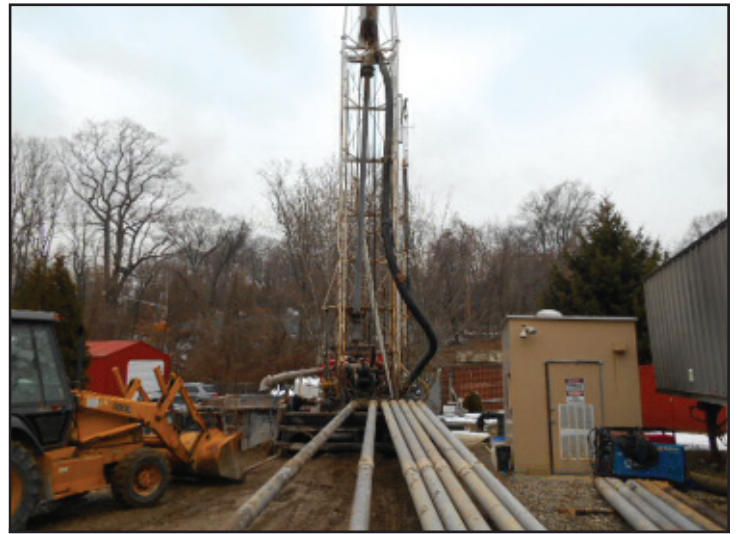
Work is underway at Well 11A, which is replacing the old well. Additionally, the wellhead is being raised to 5 feet above the ground surface to protect against flooding and flood-related service interruptions. A new well house is also being constructed to enclose the newly elevated wellhead and associated new pumping and electrical equipment.
